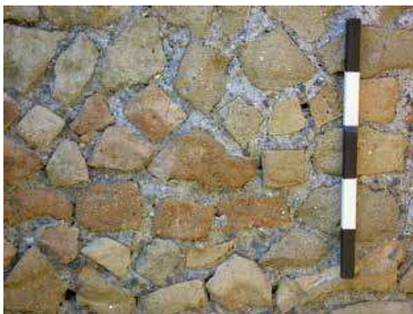
Figure 11.3d: Horrea, via degli Aurighi (III.ii.6). Rubble facing of dividing walls (photo: Janet DeLaine).
